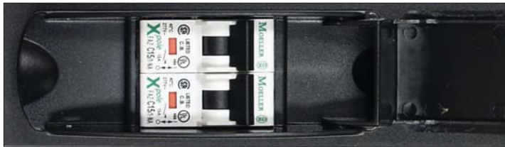
UL 489 hydraulic-magnetic circuit breaker on 30 Amp PDU.
